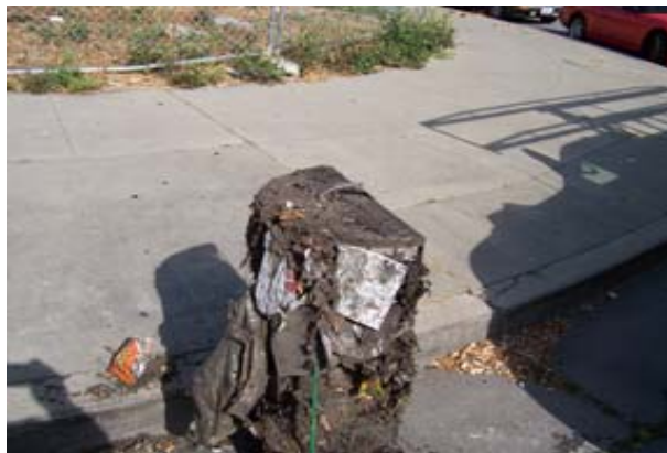
Figure 3: storm drain retrofit device clogged with plastic bags
